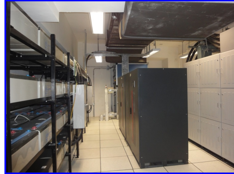
UPS and Central Battery Room (2x400kVA for Phase 1)
