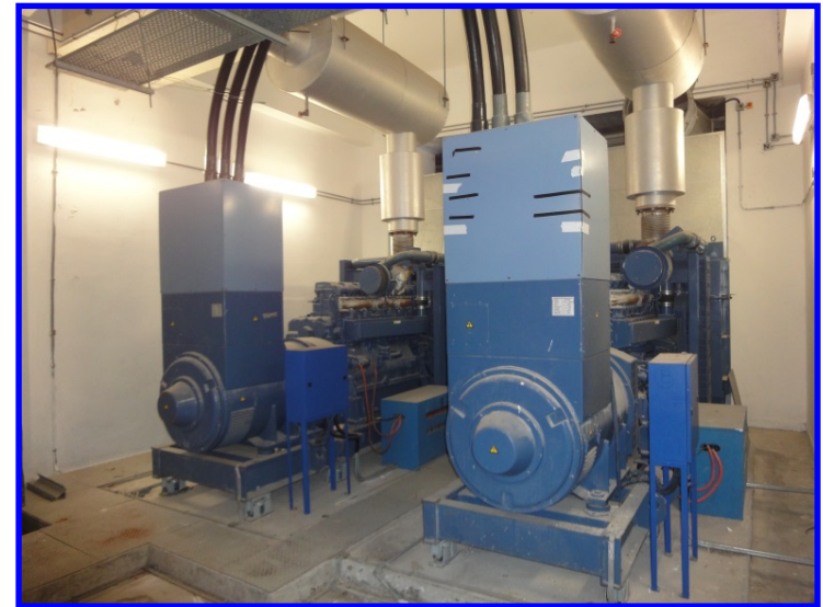
Emergency Generator (2x800kVA)
